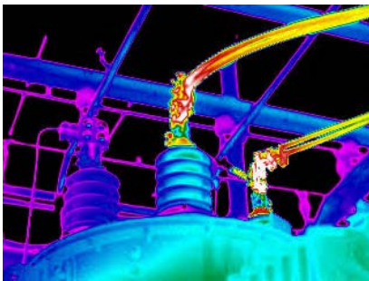
Don't Let This Thermal Condition
